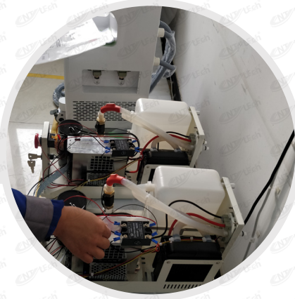
Second inspection Electrical line inspection
